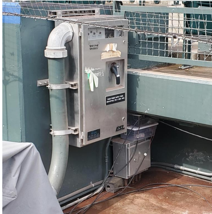
Field Level Electrical
