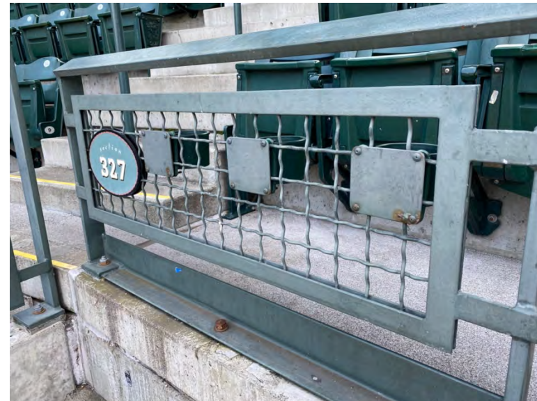
Railing at Section 327 has faded surface and showing signs of oxidation
