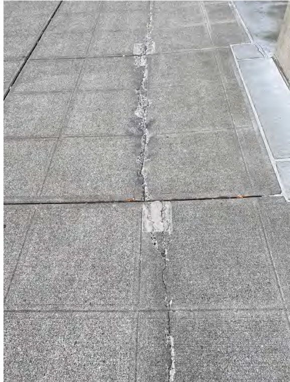
Cracking in the concrete outside the left field gate
