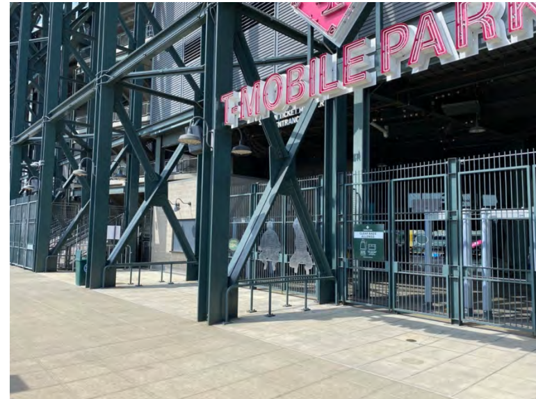
Right field gate with concrete in great condition, very little cracking - painted surfaces appear to be in good condition
