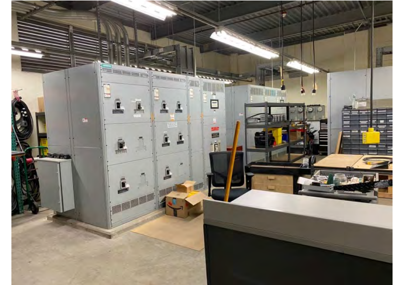
Electrical distribution room on first base side is clean, well-maintained but used as a maintenance storage area
