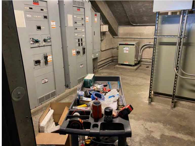
Electrical room across from Section 116 is clean but the cardboard box is a combustible material and should be removed
