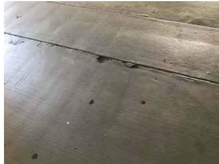
Level three of the garage is showing some concrete spalling - this is not a serious problem and is limited throughout the garage
