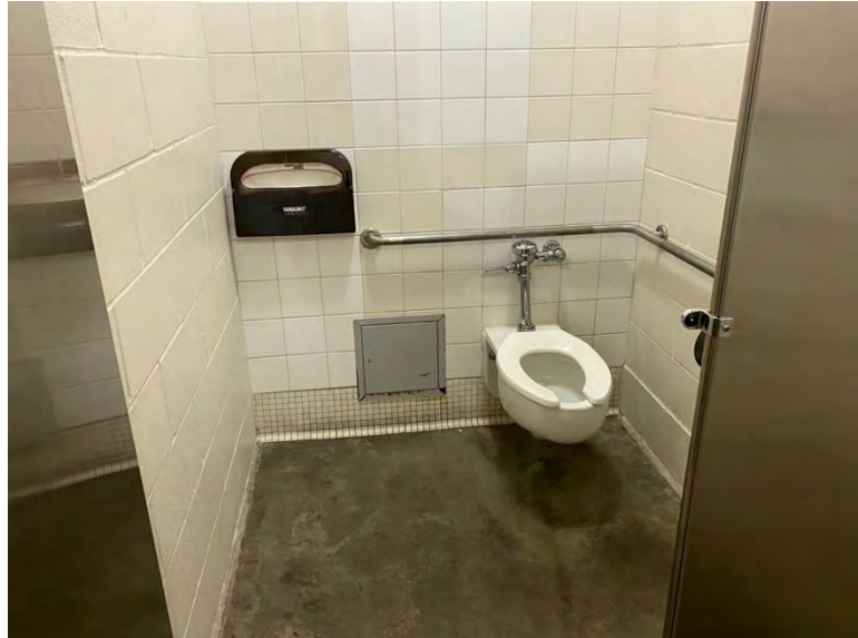
Men's restroom outside Section 150/149 is showing its age as the finishes are worn out, some broken tile, and rust on the access panel door
