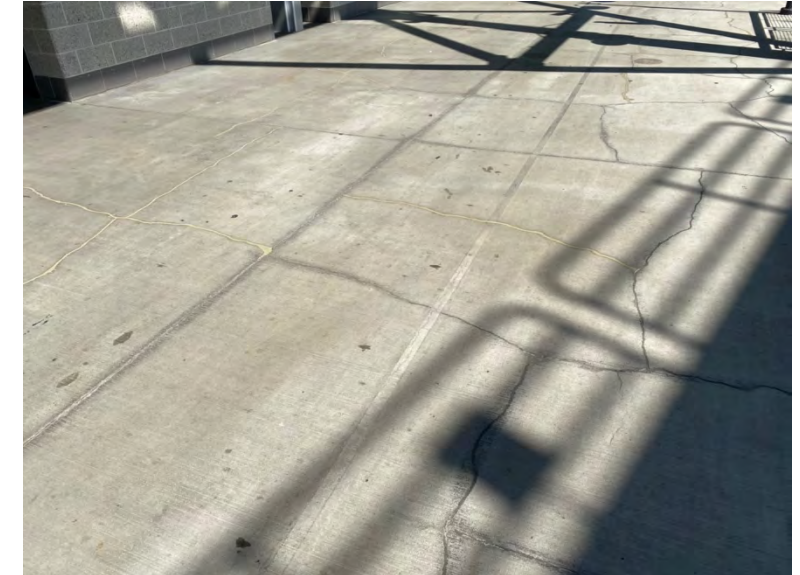
Concourse outside Section 319 was observed to have a lot of concrete cracking, but most cracks have been routed and filled with epoxy to prevent water intrusion
