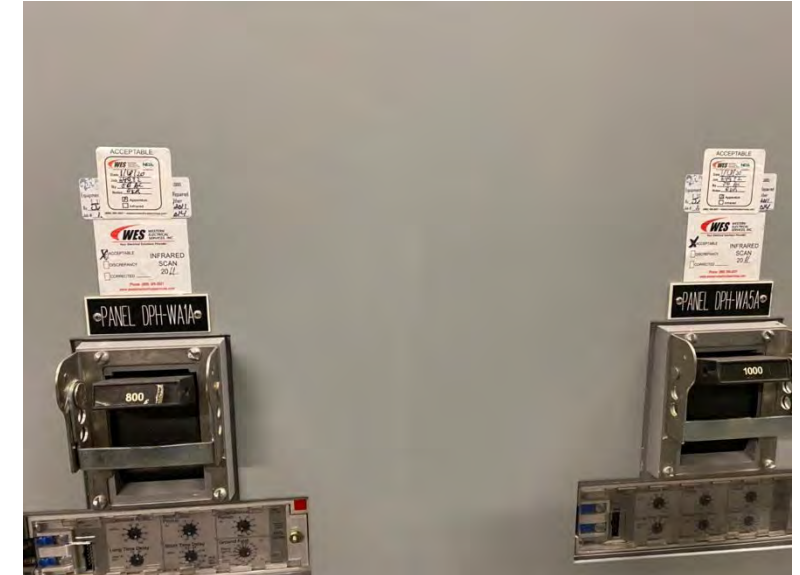
Electrical equipment was last thermal tested in 2020 and should be re-tested every 2-3 years
