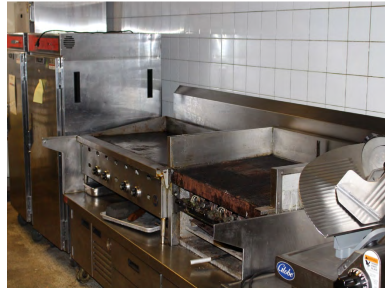
Main kitchen production line equipment is in poor condition
