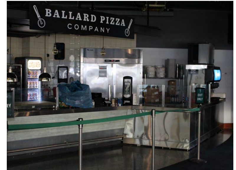
Shot of concession stand showing dinged and damaged equipment
