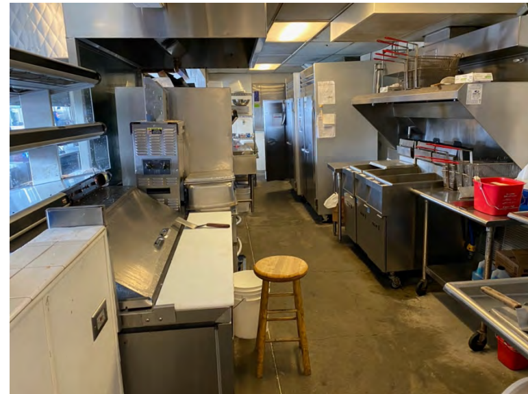
Concession stand outside Section 325 has mostly its original equipment but was observed to be clean and in good condition
