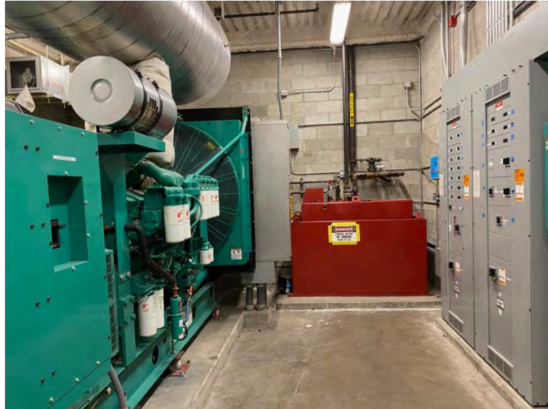
Emergency generator room was observed to be clean and equipment free
