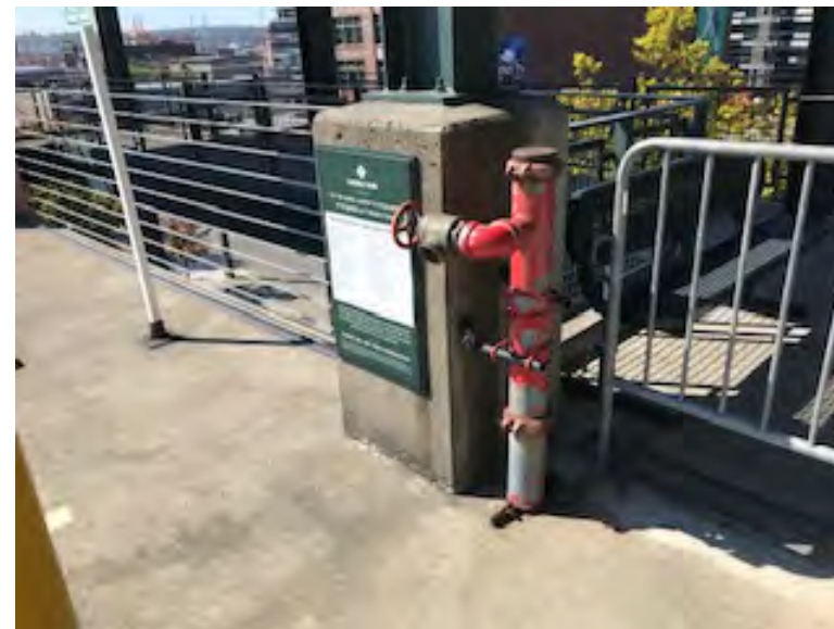
Fire connect on level six needs re-painting
