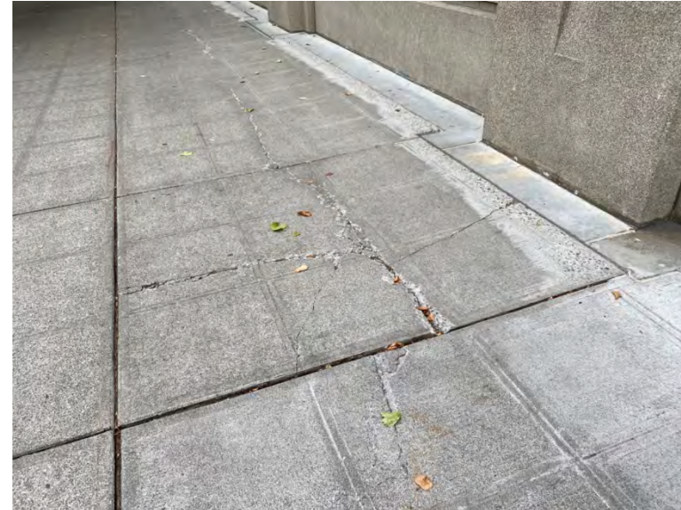
Damaged concrete outside the team store between the left field and center field gates
