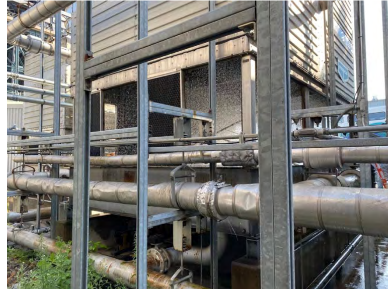
The operator is in the process of installing a new pump and a new VFD on one of the towers - the area around the towers should be cleared of vegetation
