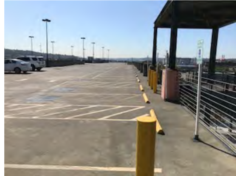
Level six looking south - concrete is in good condition and fairly clean
