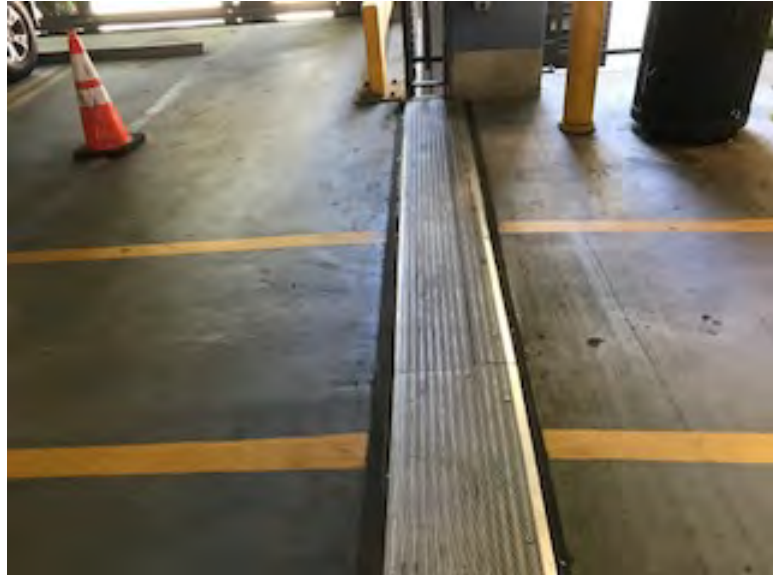
Expansion joint on level two in good condition - other expansion joints look good except for a repair on level four
