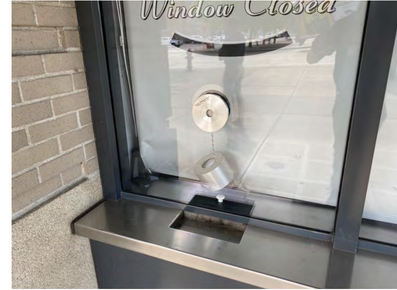
Box office window on Edgar Martinez Drive with a damaged speaker
