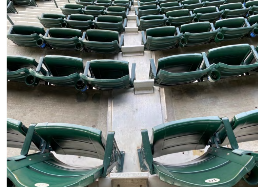
Expansion joint cover in Section 319 is in good condition as we didn't observe evidence of damage to the plate or oxidation
