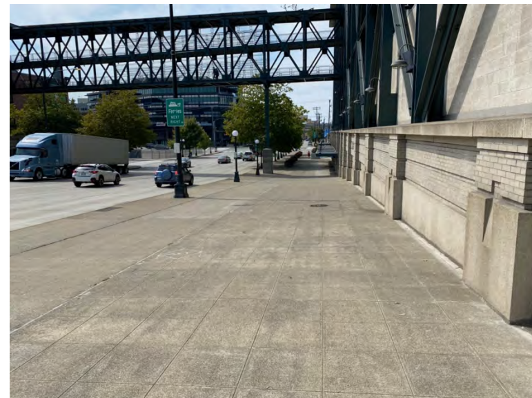
Perimeter on Edgar Martinez Drive with concrete's in good conditions and caulk joints observed to be to be intact
