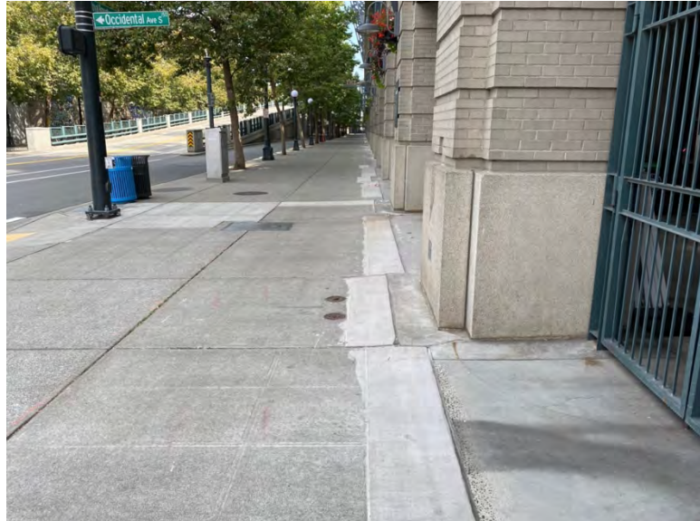
Left field gate where there has been there's been significant concrete repair due to previous subsidence
