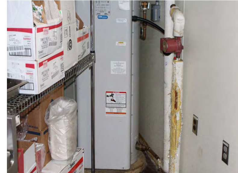
Main kitchen storage area showing damage to insulation
