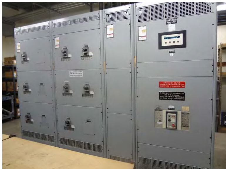
Switch gear in good condition, records show proper inspection but will need thermal testing soon
