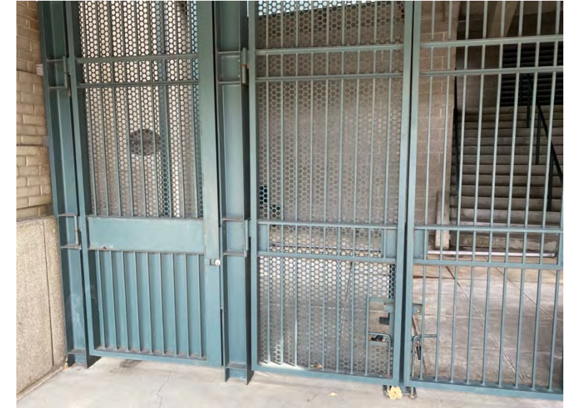
Gates at the Home plate entry was observed to be in very good condition
