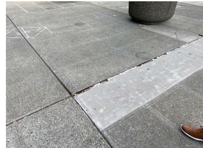
Near the BECU ATM at the home plate entrance with sidewalk subsidence creating a trip hazard
