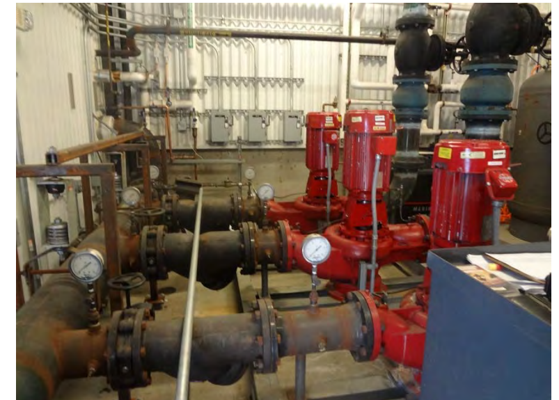
Pumps in plant area, equipment in good condition
