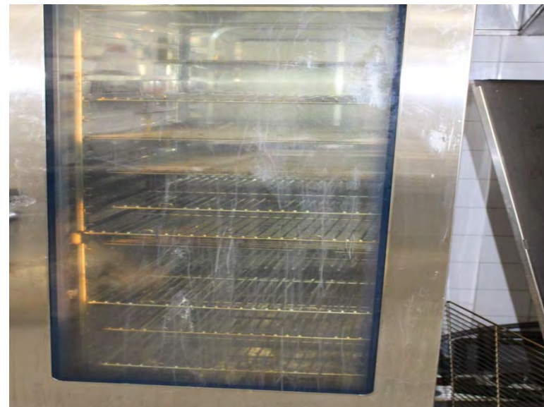
Club Level Main kitchen oven in poor condition, appears to be at the end of useful life
