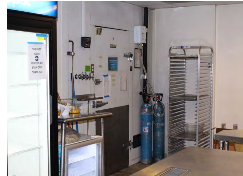
Main kitchen area was fairly clean, but gas bottles need to be secured
