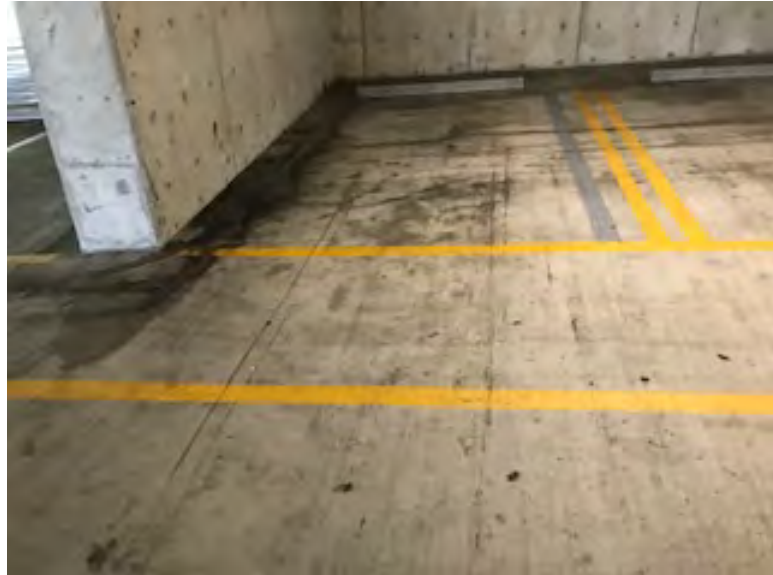
Level four showing staining and oil buildup indicating need for power washing
