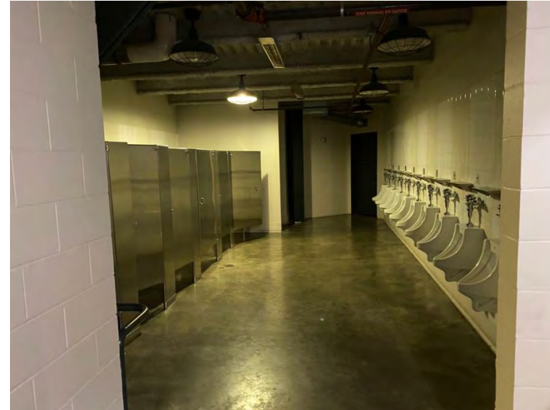
Men's restroom next to Section 112/114 with metal partitions in very good condition
