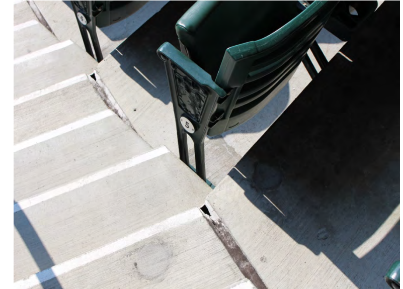
Breakup of caulking joint
