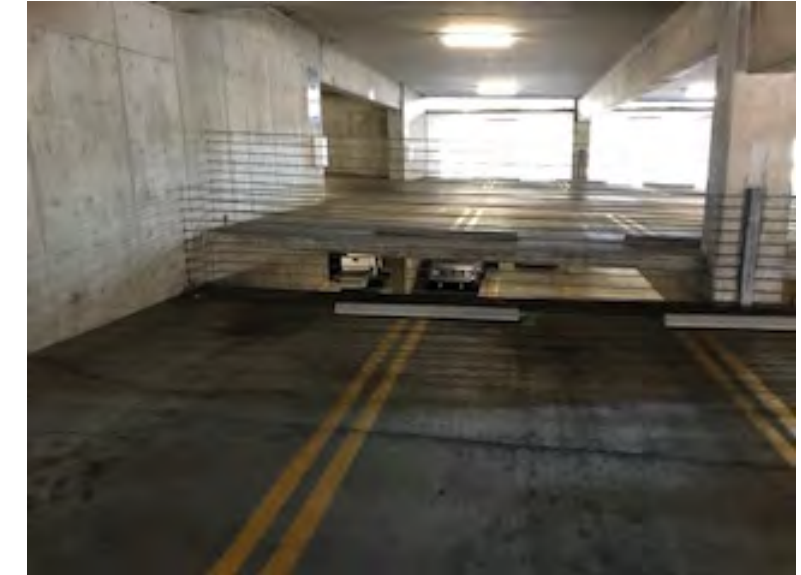
Level three showing strong dirt and oil buildup
