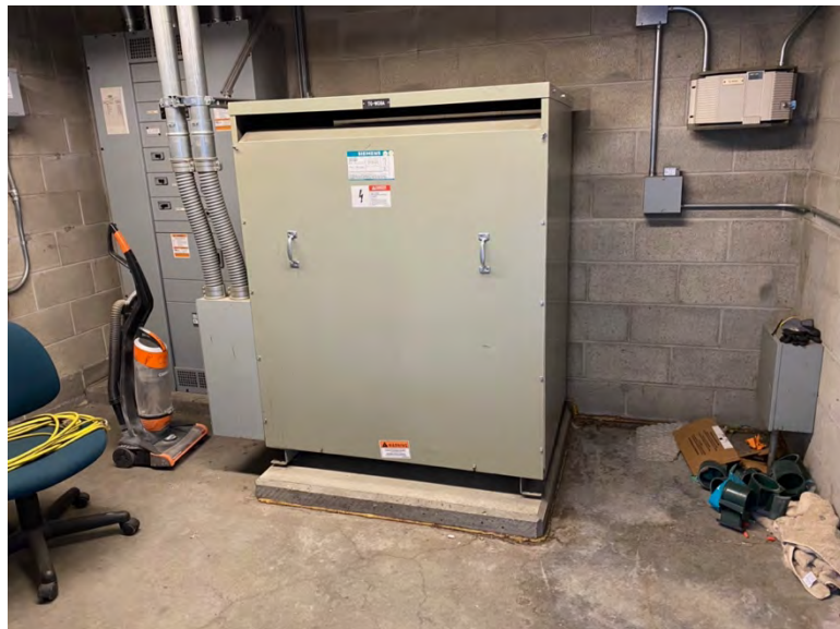
Electrical room outside section 345/344 has some debris and used as a storage area for seat parts - this electrical room also has a transformer that has a high pitch hum that seems to be louder than normal
