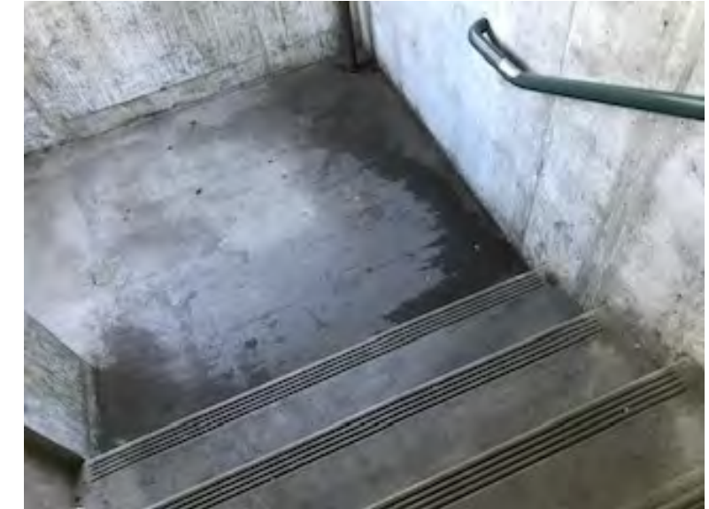
Stairway on north end leading down to level three is stained and needs cleaning
