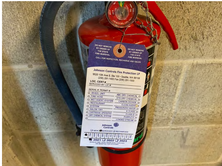
Fire extinguisher in Section 309/310 electrical closet has an up-to-date inspection
