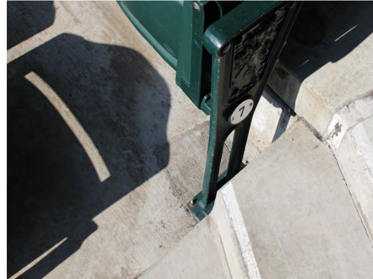
Seat end cap showing some corrosion. Seat anchors are still in good condition here
