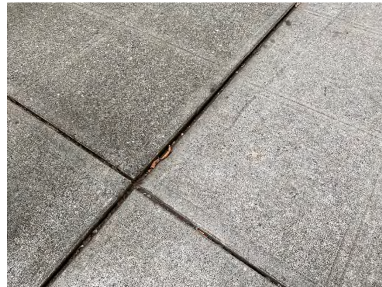
Concrete that has subsided creating a potential trip hazard between left field and center field gates
