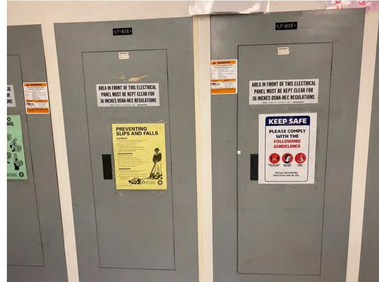
Electrical panelboards in Diamond Club kitchen with signage warning area in front of the panels should be free of obstructions
