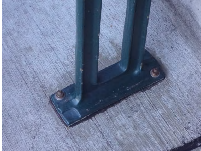
Seat standard in 100 level, section 127 in good condition with minimal rust on attachment bolt – seating replacement should involve the installation of stainless-steel anchor bolts
