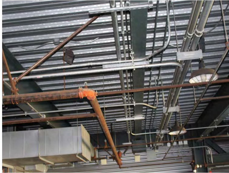
Rusted pipes but no sign of leakage
