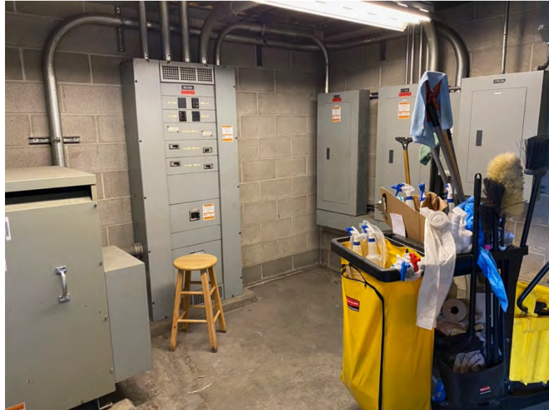
Electrical room in Section 309/310 vomitory used to store housekeeping cart – these items should be stored in janitor’s closets
