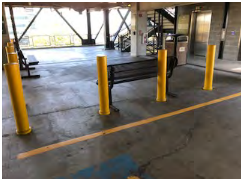
Level five showing elevator landing area was clean, but cracking is noted on floor area
