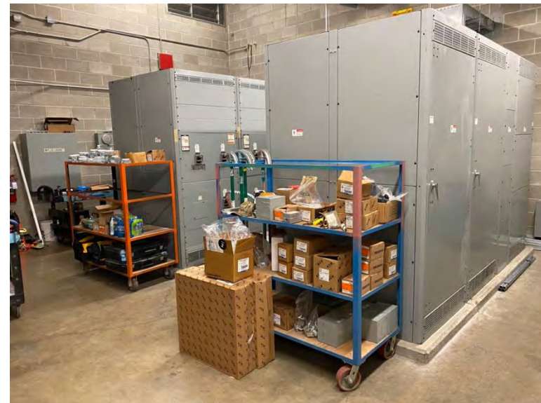
Main electrical room on 3 rd base side is clean but used for parts storage
