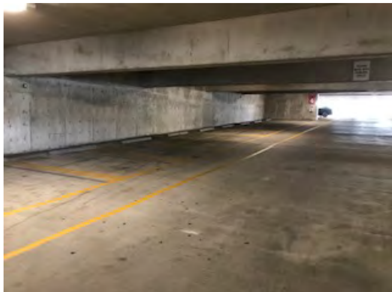
Level three headed towards level four on the south side the floor, walls, and ceiling in good condition - signage and wayfinding in the garage is somewhat confusing
