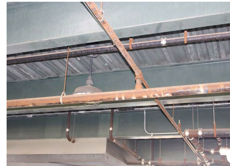
Overhead pipes with considerable rust
