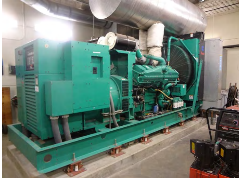
Emergency generator in very good condition, generator is test run regularly
