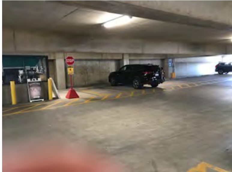
2 nd floor of garage, concrete is in good condition but needs power washing
