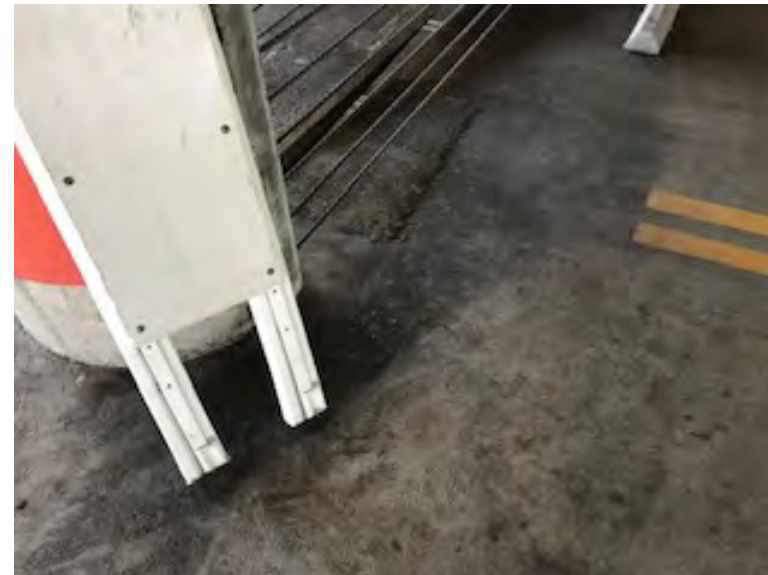
Level four showing dirt and oil buildup that needs cleaning
