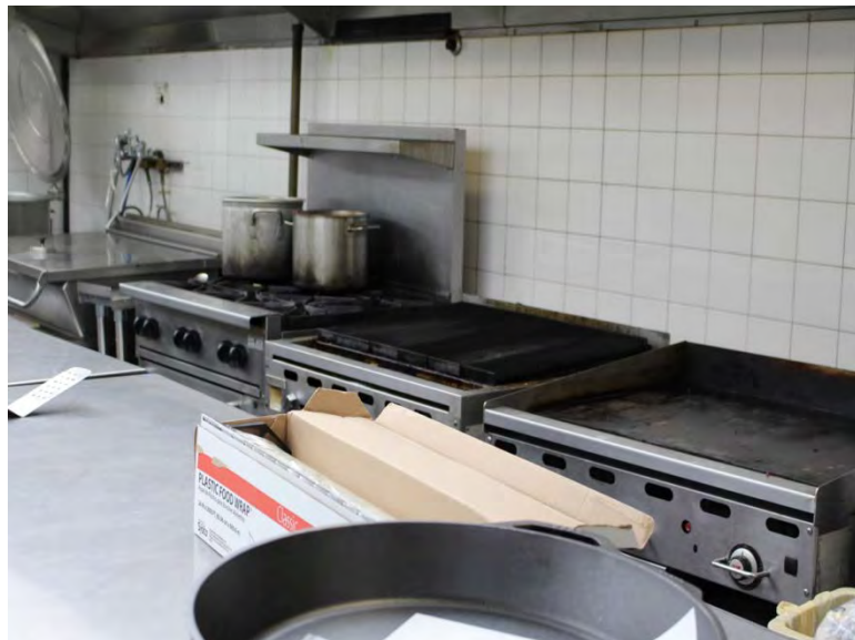
Main kitchen hot line equipment is showing wear
