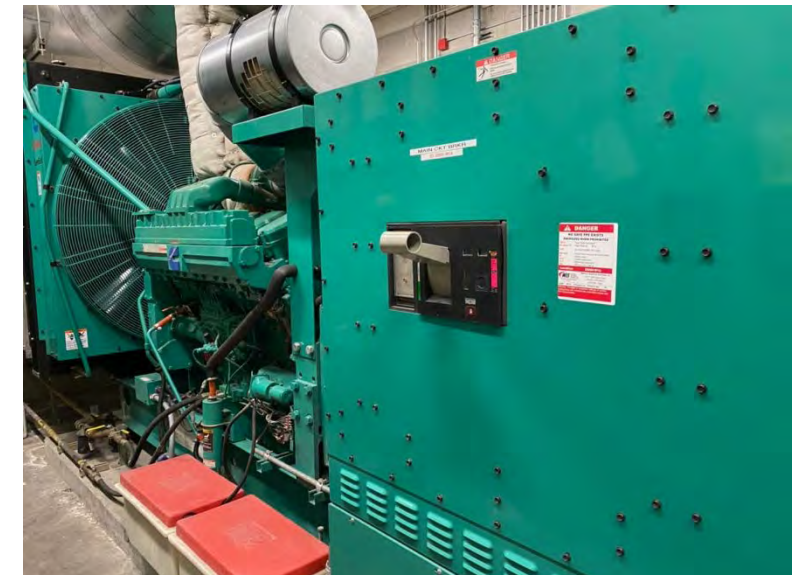
Emergency generator is exercised regularly
