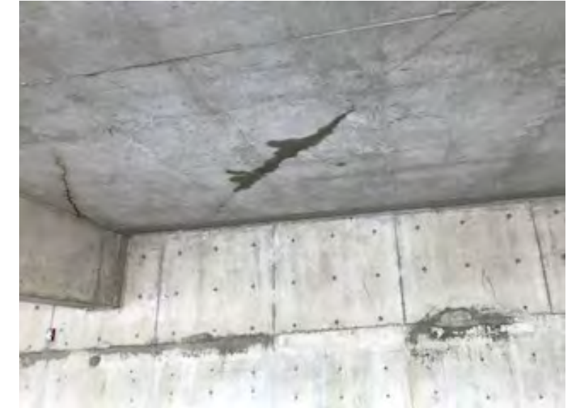
Ceiling on level three showing cracking in concrete and water intrusion
