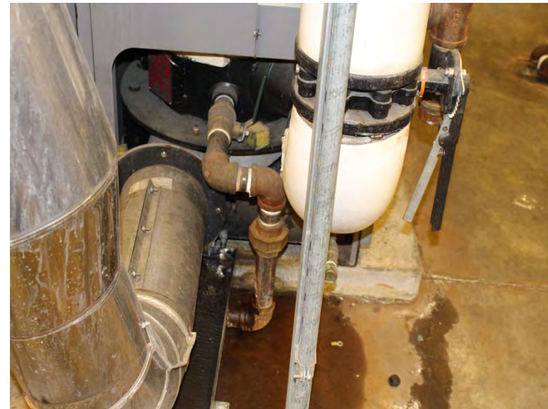
Hot water boiler showing rust and previous leakage, plant floor should be sealed with epoxy
