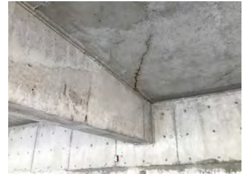
Same area on level three, looking west - water intrusion and cracks that need attention
