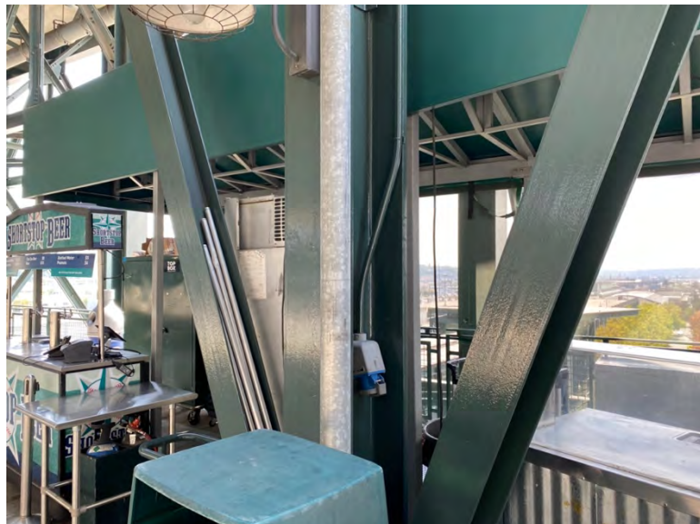
Concourse outside section 327 the structural steel appears to have been recoated recently and was observed to be in very good condition
