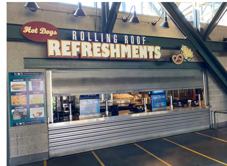
Concession stand outside Section 127 with branding in fairly good condition with countertops and the metal corrugated panels below having a few dents
