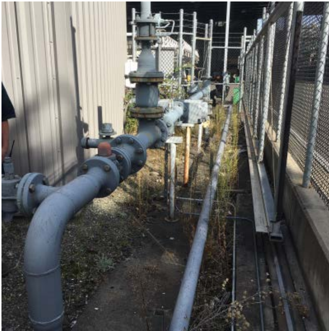
Natural Gas Line Provided with SGSV
