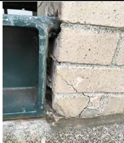
Beam end with failure at brick pilaster.
