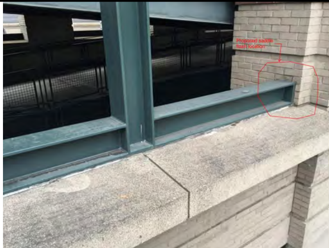
Condition prior to saddle flash install and sealant replacement.
