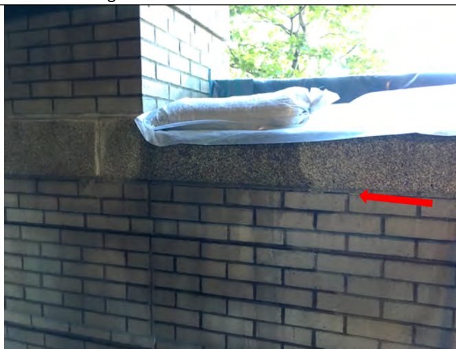
Water infiltration at brick wall to cornice joint during isolation water test.
