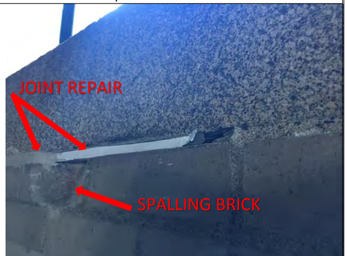
Brick wall to cornice joint repair in progress, located at cornice associated to the west facade saddle flash installation. Also note failure of joint causing spalling brick.
